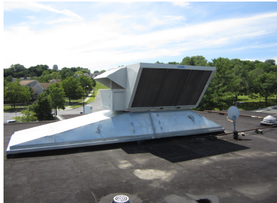
Downsized Rooftop Unit on Existing Roof Curb
